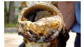
Grease-choked sewer interior
